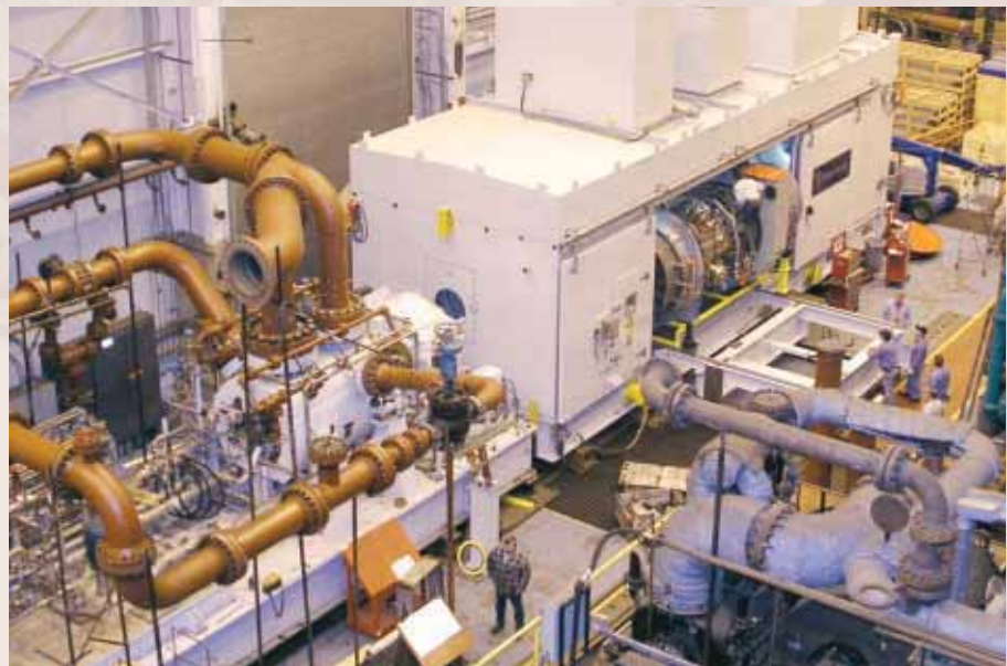
Trent 60 engine on test, driving a centrifugal compressor at full load.
